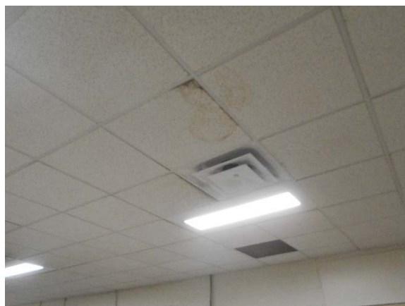
Portion of Affected Area in Room 133
