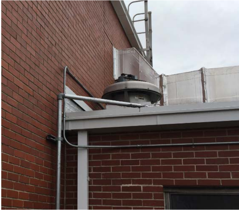
Figure 31 Kitchen exhaust fan out of service
