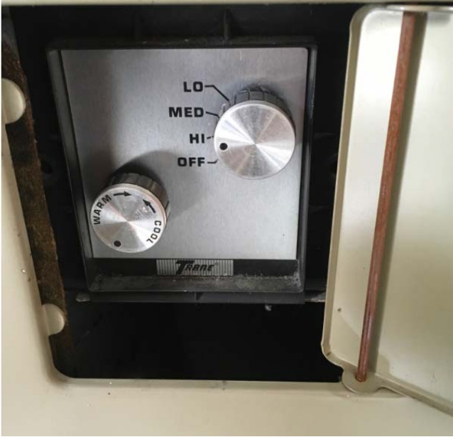
Figure 23 Hot Water Cabinet Unit Heater controls
