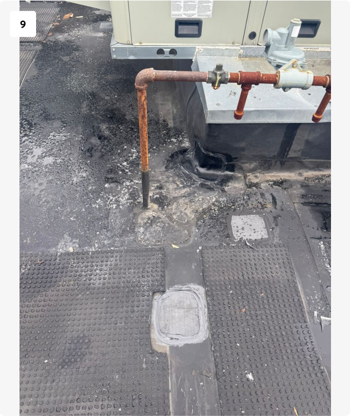
Project: 815866 US Army Reserve Center AMSA ROOF LEAK Date: 12/5/2024, 11:17am Creator: Matthew Mullins
