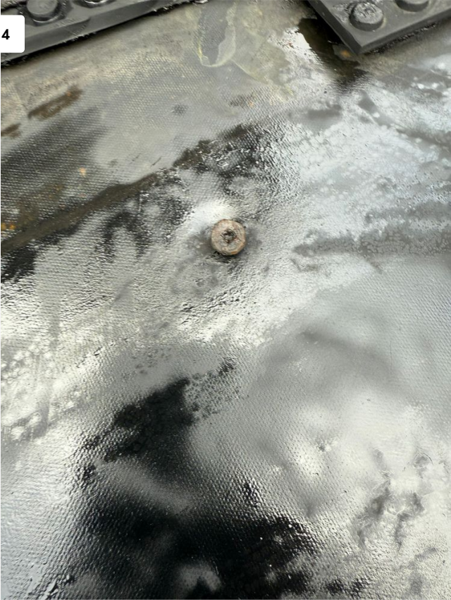
Project: 815866 US Army Reserve Center AMSA ROOF LEAK Date: 12/5/2024, 11:04am Creator: Matthew Mullins
