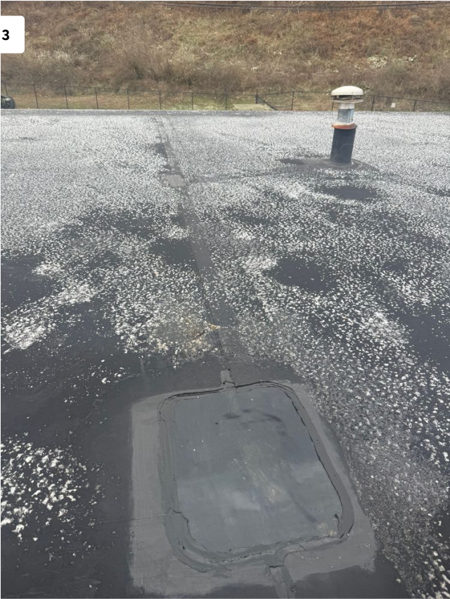
Project: 815866 US Army Reserve Center AMSA ROOF LEAK Date: 12/5/2024, 10:31am Creator: Matthew Mullins
