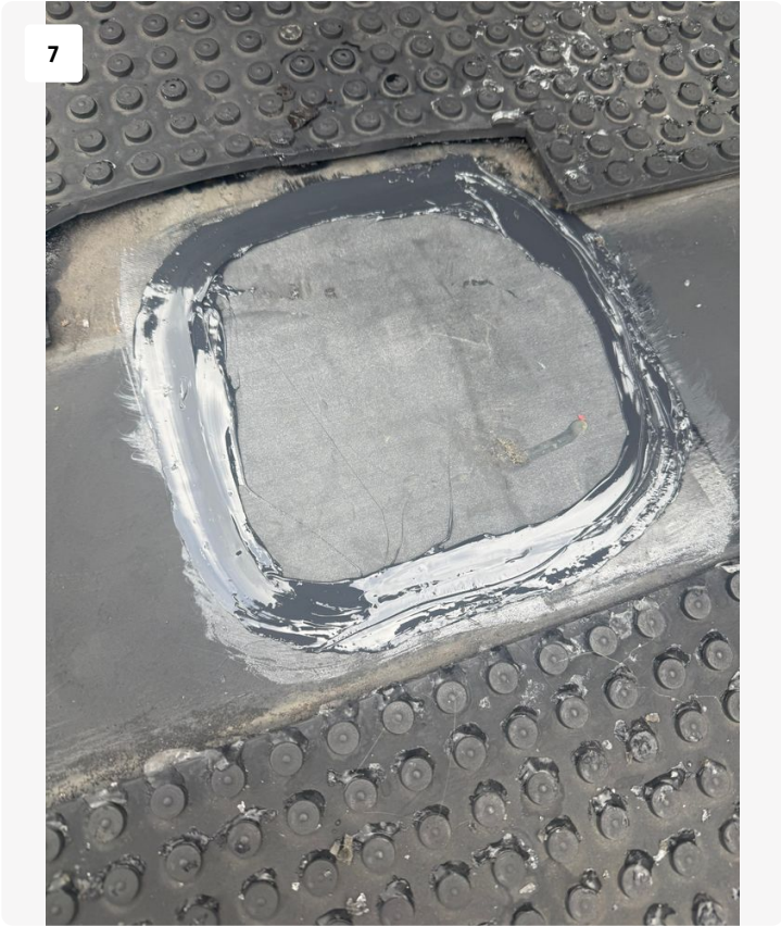
Project: 815866 US Army Reserve Center AMSA ROOF LEAK Date: 12/5/2024, 11:14am Creator: Matthew Mullins
