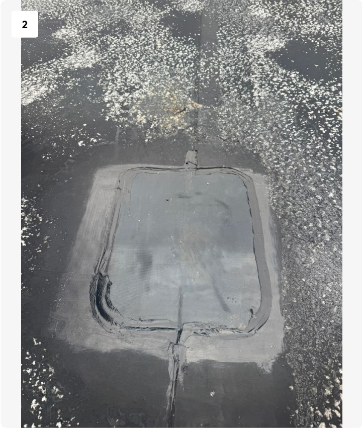
Project: 815866 US Army Reserve Center AMSA ROOF LEAK Date: 12/5/2024, 10:31am Creator: Matthew Mullins
