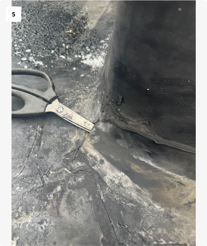
Project: 815866 US Army Reserve Center AMSA ROOF LEAK Date: 12/5/2024, 11:04am Creator: Matthew Mullins
