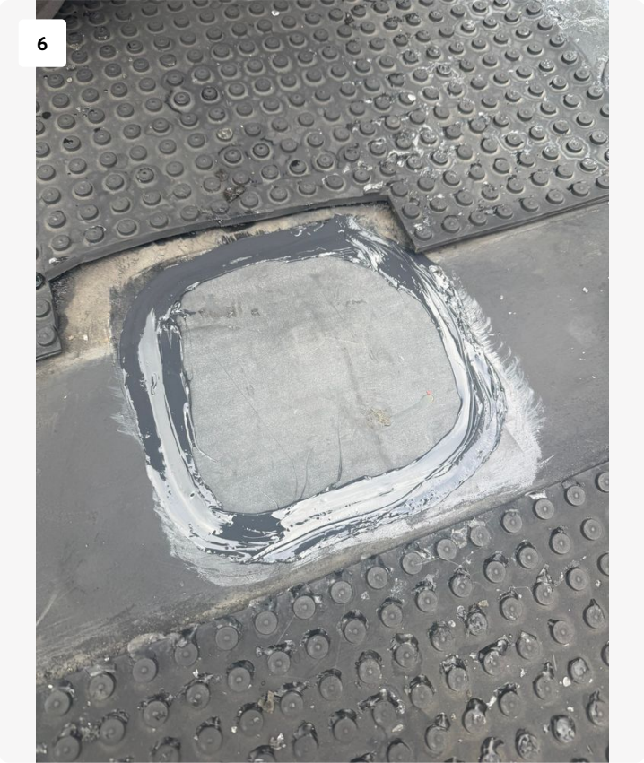
Project: 815866 US Army Reserve Center AMSA ROOF LEAK Date: 12/5/2024, 11:13am Creator: Matthew Mullins
